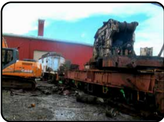
With the boom and pulleys and cab removed, December 30, 2022, only the gear box was left on base of the car.
