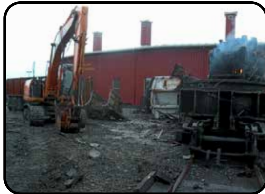
Gear box covering removed, laying by digger, boom car body laying on it side, workmen torching the gears. January 17, 2023
