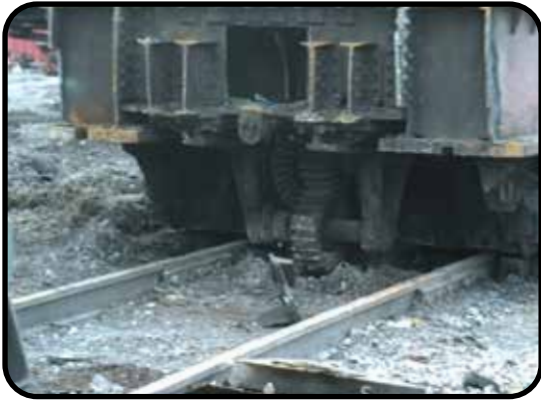
Close up of center power truck gears used to transmit power to end trucks. January 24, 2023
