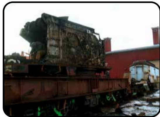
Workmen torching the gear assembly into small parts, December 30, 2022, to remove from the base of the car.
