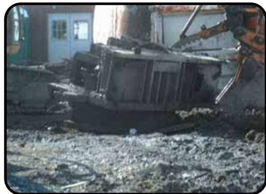
Ring gear removed, leaving only the base piece to be cut up. February 2, 2023 Still a heavy thick piece needing to be cut up to be able to haul it.
