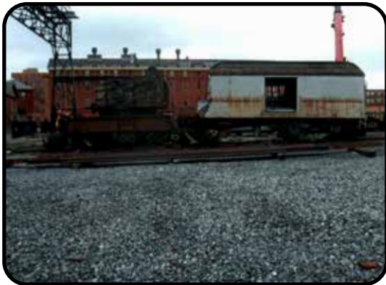
With the frame cut off the boom, car body is moved closer to get the tracks off. January 13, 2023
