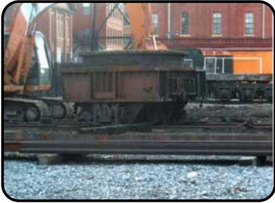
End power trucks removed, only center power truck and crane pivot base remain. January 24, 2023
